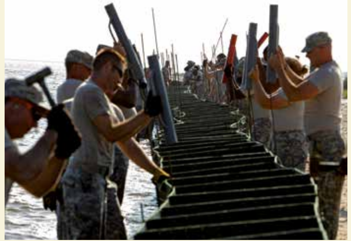
1.37 > Barriers were erected in a futile attempt to protect Dauphin Island.
